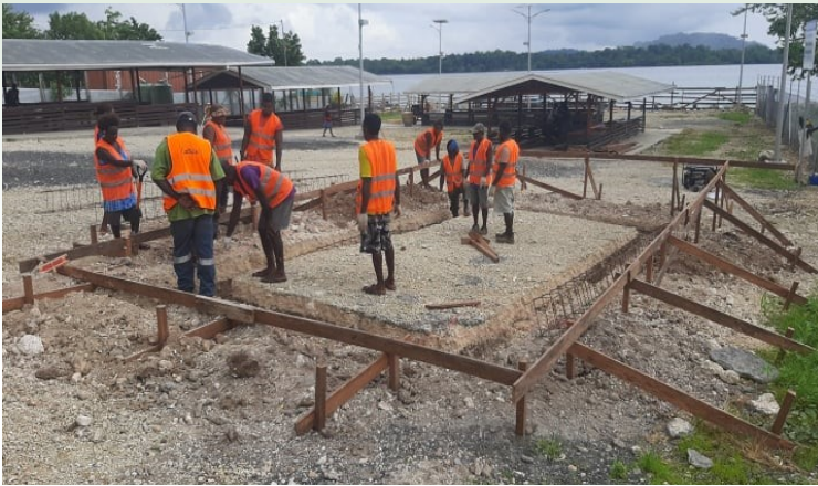
Work on the Noro market ablation block has started this week. Currently workers are working on the foundation by next week structures should be up to follow by other stages.
