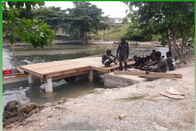
The Nusatupe jetty is in the final stage of completion this afternoon. So far 95% of the job is completed.
