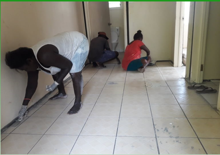
Full completion of tiling in the Nusatupe quarantine centre building will be next week. Currently local workers are working hard to catch up with the timeline.
