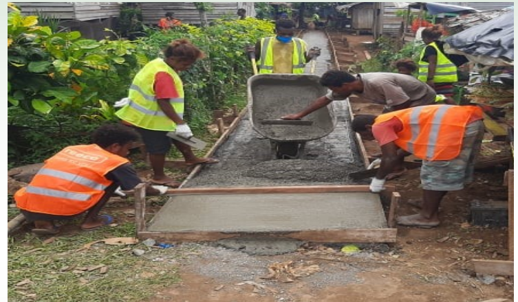
Second footpath is progressing well at the moment in Mobil area of Noro. The new footpath is an extension to an old one that completed some months ago. With this new one it will make life easy for the people living in this crowded areas.
