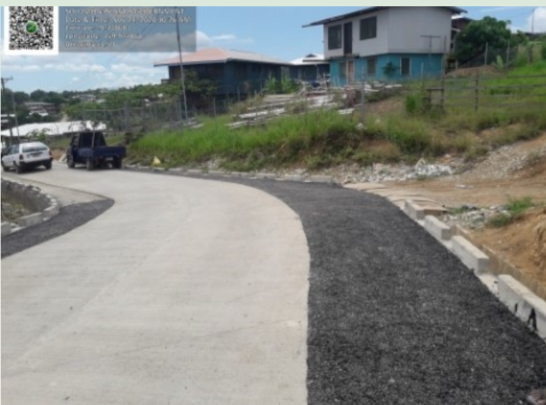
Work on the Kombivatu, feraladoa, Ferakusia, Matariu road has reached 80 percent of job done. The additional tar of the road makes the road perfect to withstand running water which usually block the drainage system.
