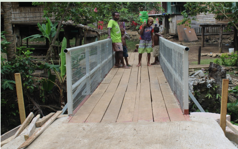
The newly completed footbridge at Botanical garden in central Honiara is been described by the community as life saving vehicle. Yesterday a young boy carrying a bag of food to their house said had it not the bridge he will certainly go down the filthy creek to cross over.
