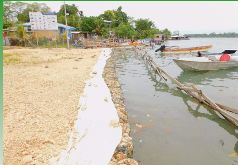
Work on the preparation of Noro market jetty is progressing very well at Noro. Already filling up of gabion basket has completed team is now waiting for commencement of constructing the new jetty.
