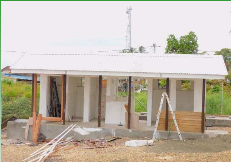
Final touches on the completion of Noro ablation block is shaping up very well. Full completion will be around end of March.
