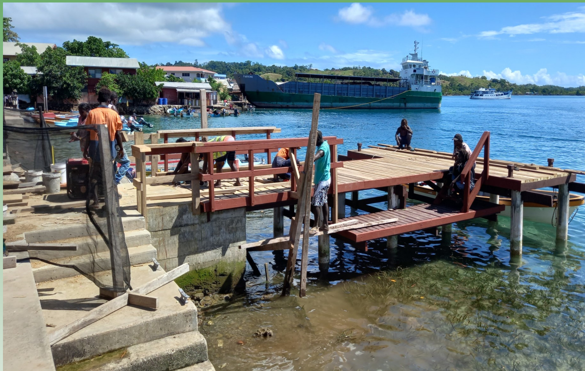
Gizo Market jetty is in the final completion stage. Currently, workers are working on the final touches and finishing jobs. Full completion is expected at the end of this month.
