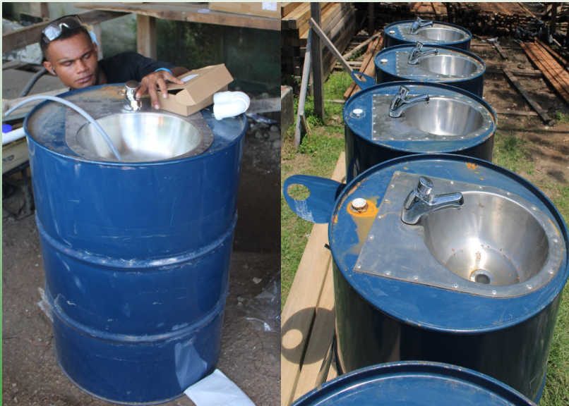
Work is currently underway in Honiara PMU on the installation of hand washing sink. The sink once completed will be distributed to schools and clinics in Honiara as part of the covid prevention measures.
