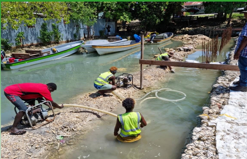
Work on the Munda seawall protection is continuing despite the big challenge draining out of water in foundation area. This week workers work on the third segment on the installation of foundation work and concrete pouring.
