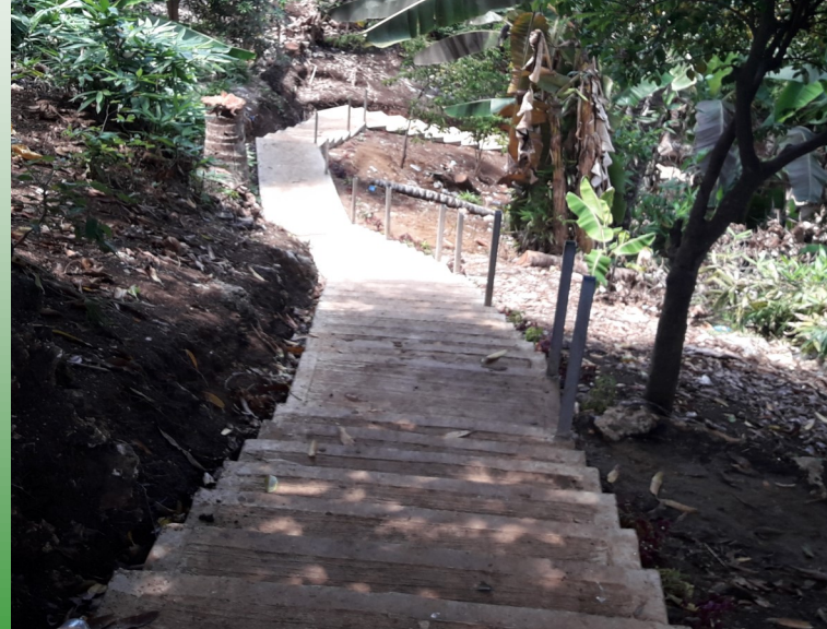
Work on Jericho Jacob's ladder in East Honiara is progressing well. Expecting to reach final section over the coming days.
