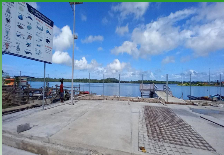
The Noro fish market finally completed. Workers are now working on fencing the area and do a cleaning up. The market will be commission and handed over to the Western Provincial government soon.
