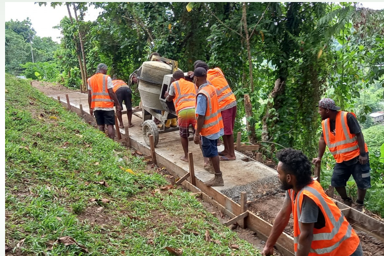
The Jacob's ladder at Auki tophill is progressing well. Already it reaches the middle section. Work is continuing.
