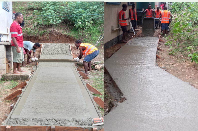
Work on new footpath at Mbokona clinic of Central Honiara has commenced this week. Work is continuing and is expected to complete in the coming weeks.
