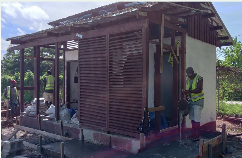
The JF Kennedy ablution block in Gizo is progressing well. In the coming weeks workers will install toilet bowl and other amenities.
