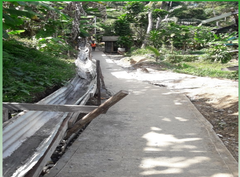
The new footpath at Vara creek is soon to complete. Currently workers are working on completing the last section and on to railing.
