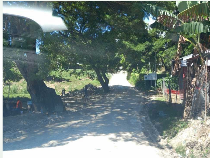
Work on the climate resilience road in the Kukum Tanuli will resume in the coming weeks. The contractor is waiting testing with MID and they will mobilise to do form work thereafter.
