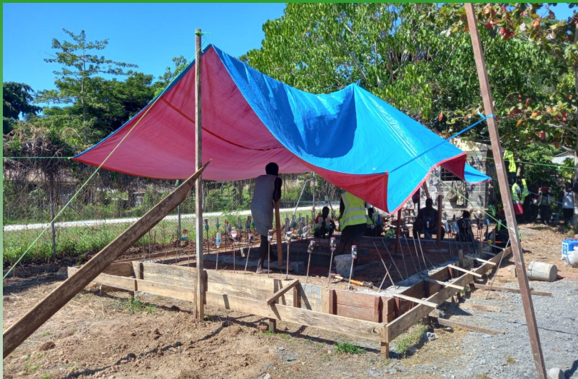
Work on the ablution block at the JF Kennedy stadium in Gizo is progressing well. Foundation work has been completed now they move on the stage.
