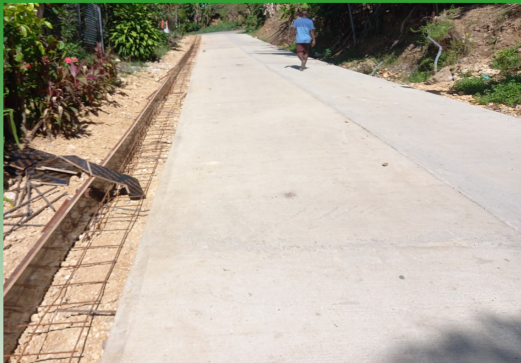
Work on the drainage on the recently completed roads in Chipuchao, Lai and Tehamurina in the central Honiara is ongoing. There will be proper drainage systems on these new concreted roads to allow water to flow freely during bad weathers.
