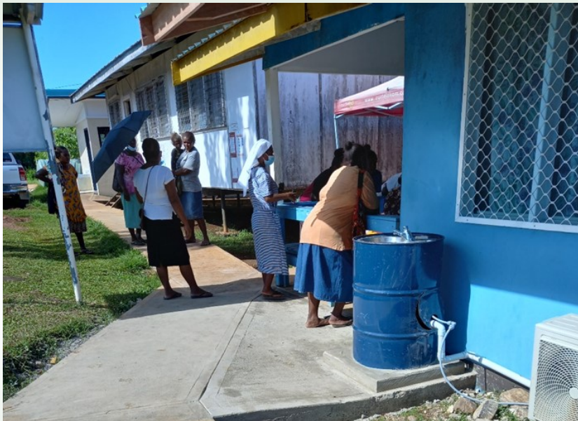
The newly installed wash station at Kiluufi hospital is now in use. Patients acknowledge and thanked the project for facilities as it helps them a lot whilst in the hospital area.
