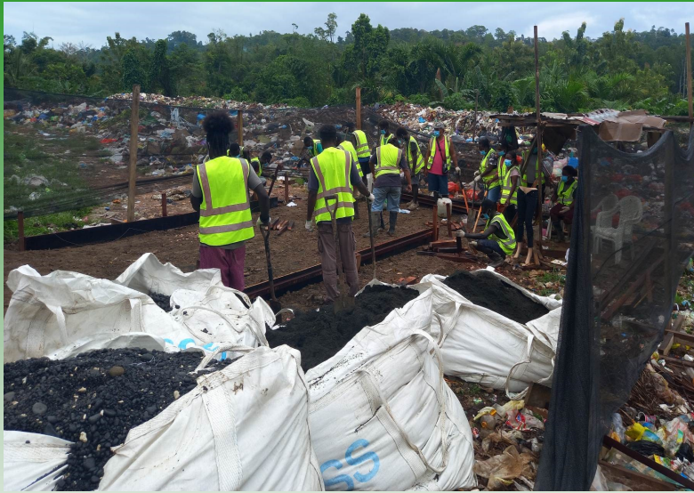
Work on component 2 at the dumpsite in Gizo is going on well. Currently workers are working on back filling.
