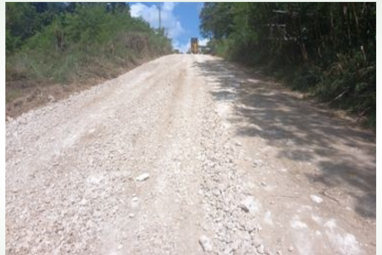
Rehabilitation of Barana road above the borderline area in Honiara is currently going well by Hitech company.
