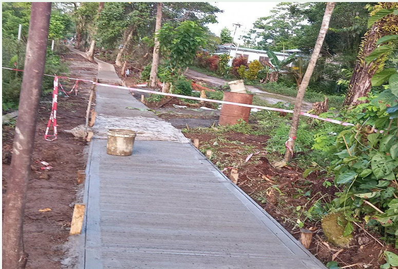
The small Baru footpath at Noro is near completion. There are few more sections to be slab then the footpath should be fully completed.
