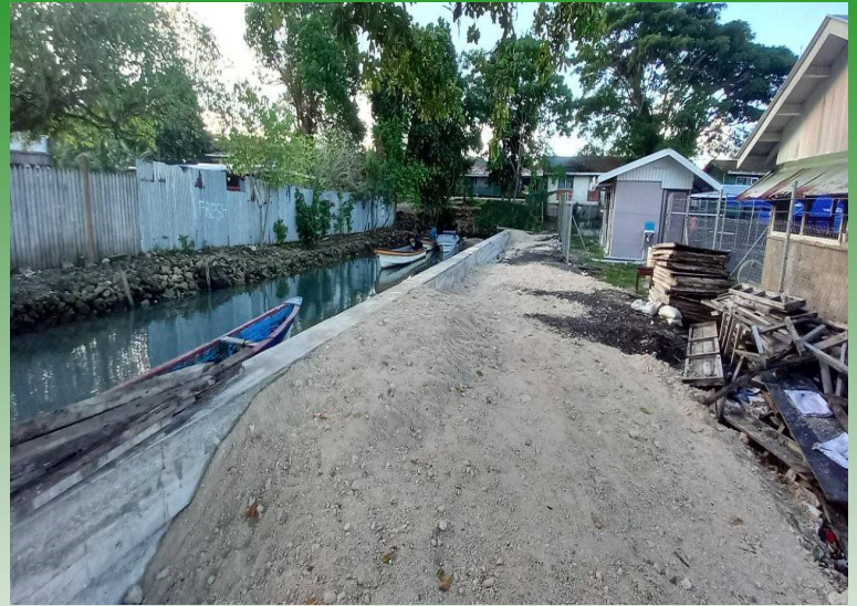
Work is currently going on the backfilling the completed Munda seawall. The shoreline protection wall has completed and so far boat enjoying berthing along the wall.
