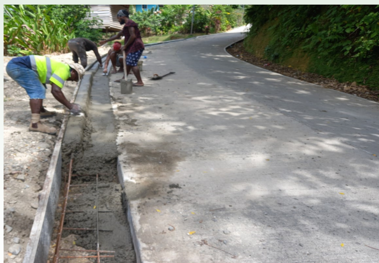
Work on drainage system on the newly climate resilience roads at central Honiara is going on well.
