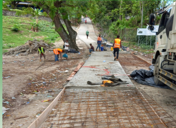
Work on the climate resilient road at Tanuli is progressing well. The concrete road runs from Kukum field up to the steep section.
