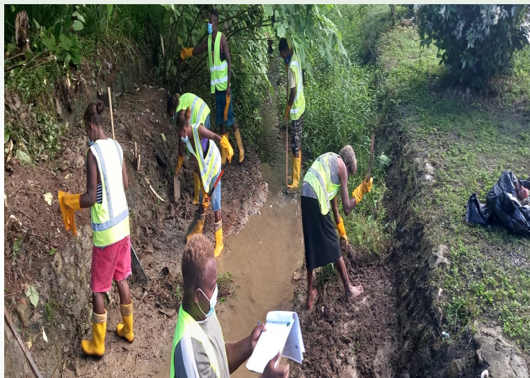
A group is currently cleaning up the drainage at Kunu in Auki. The drainage needs to be clean every time to keep the water running. Kunu is one of the community that benefited from the project. Next week their footpath towards the water source will be commission and handed over to them.
