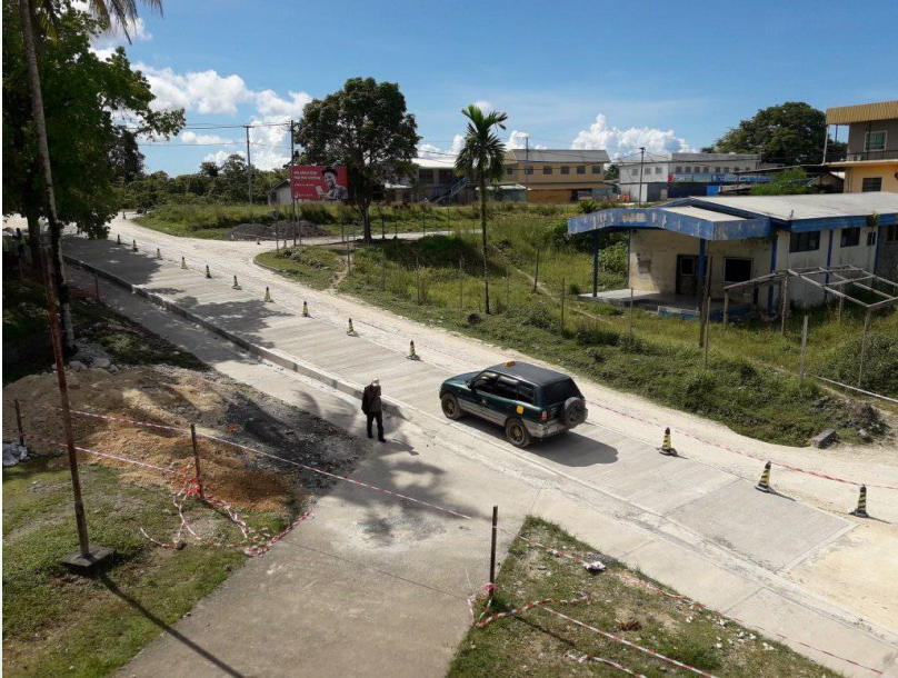
The first lane of Noro concrete road has been completed and open for public use yesterday. The new concrete has been describe by many as a blessing for Noro CBD. Meanwhile work on the second lane has been started.
