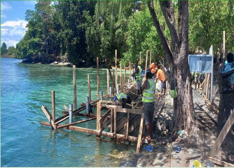
The Nusatupe jetty is progressing well. Currently workers are working on casing the concrete part of the jetty. Soon they will work on installing the bearer and flooring.
