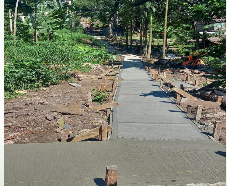
The Unafi footpath in Auki will be complete by next week. Only last section is left to complete follow by cleaning up.
