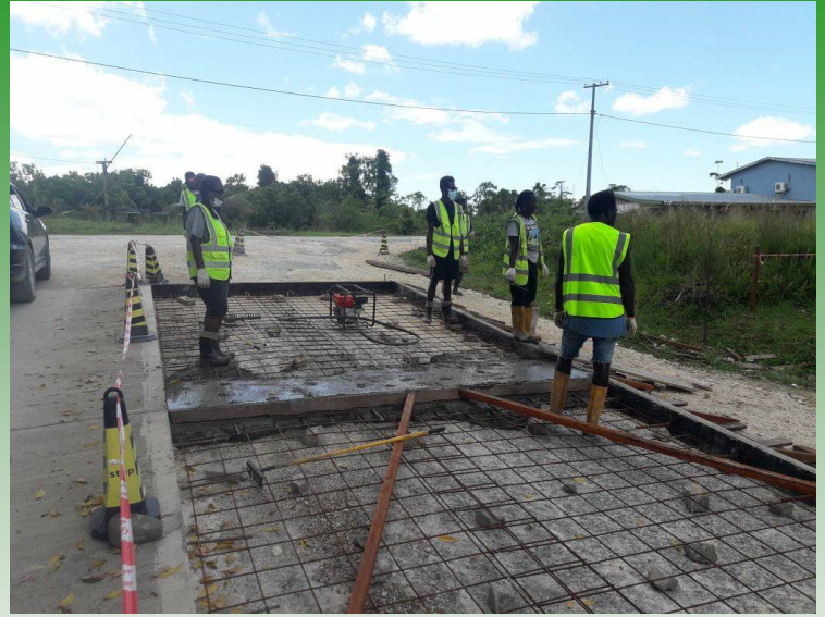
Work on the second lane of the Noro concrete road is progressing well. Slabbing of the first section is going on and will continue next week until complete then will work on the drainage system.
