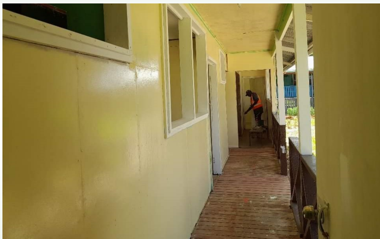
The refurbishment of Noro Clinic is progressing well into the finishing stage. Currently workers are doing final touches and soon the work will complete.
