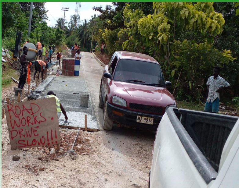
The concreting of second lane in the Gizo Top Hill road is soon to complete. Most people up the Top Hill area are already excited on the new development which help the residents up the hill.
