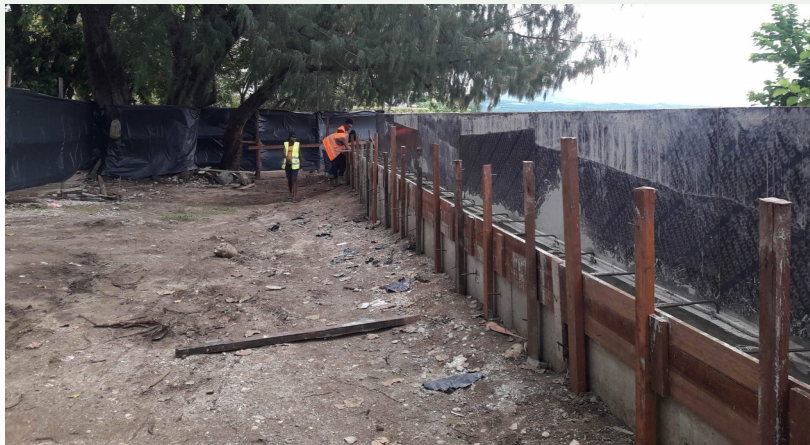
Work on the children's park shoreline protection is going on very well. So far the workers completed the first casing and they are moving on to the next one.
