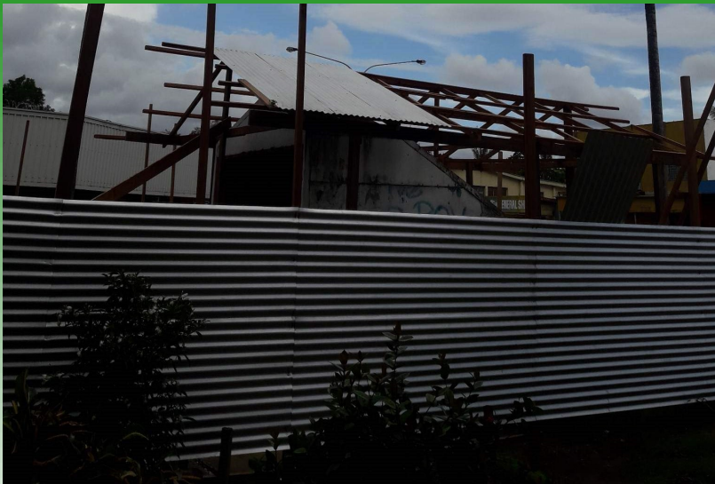
A temporary shelter at the Point Cruz under pass is shaping up. This afternoon the workers put up the roofing to protect underpass from rain while work continues inside.
