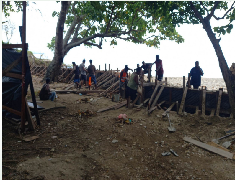
The concrete pouring at Childrens park wall has been completed. In the coming weeks workers will work on the next phase of the project
