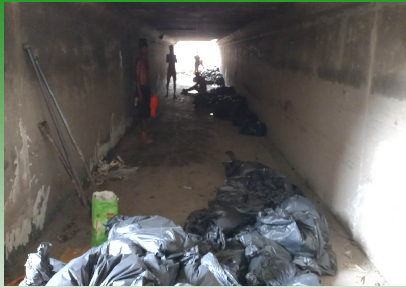
Cleaning up in the Point Cruz under pass has been completed. Next stage will be working on the improvement on the surface.
