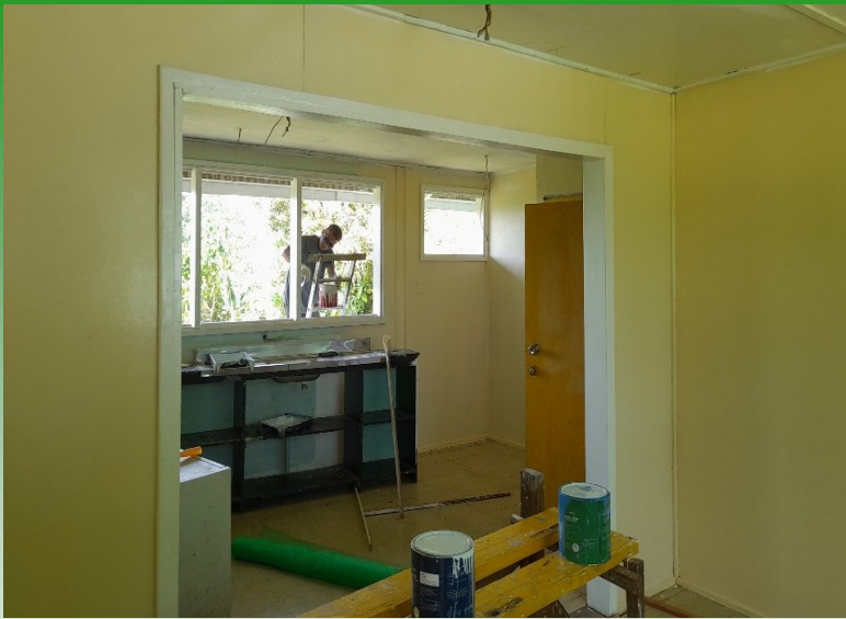
Work on the Noro clinic is in the finishing stage. Currently painting is going on to be follow by cleaning up.
