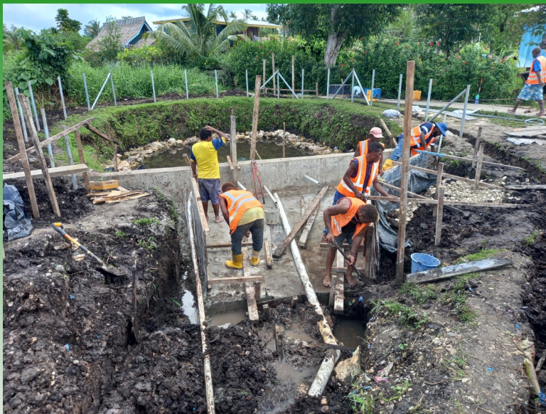
Work on securing and improving the Kunu water source in Auki is progressing well. The water source is the main source for the residents living around the Kunu catchment area
