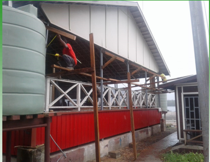
Work on the phase two of MSG building has started. This will continue in the coming weeks.
