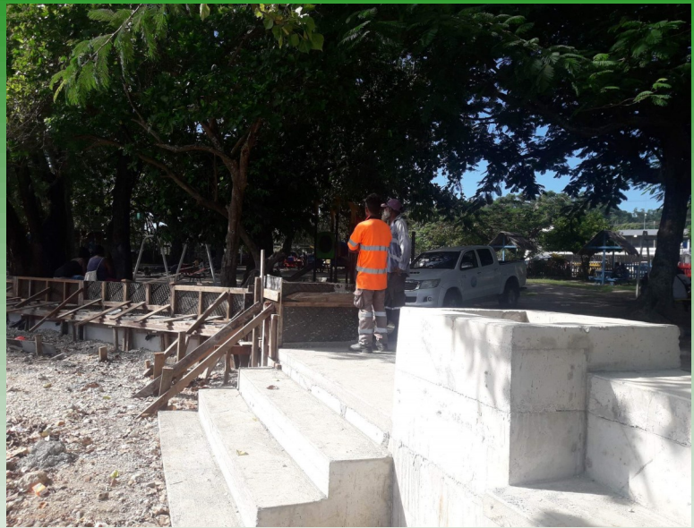
The children's park upgrade is completed. In the coming weeks the office boys will work on the back filling the area.
