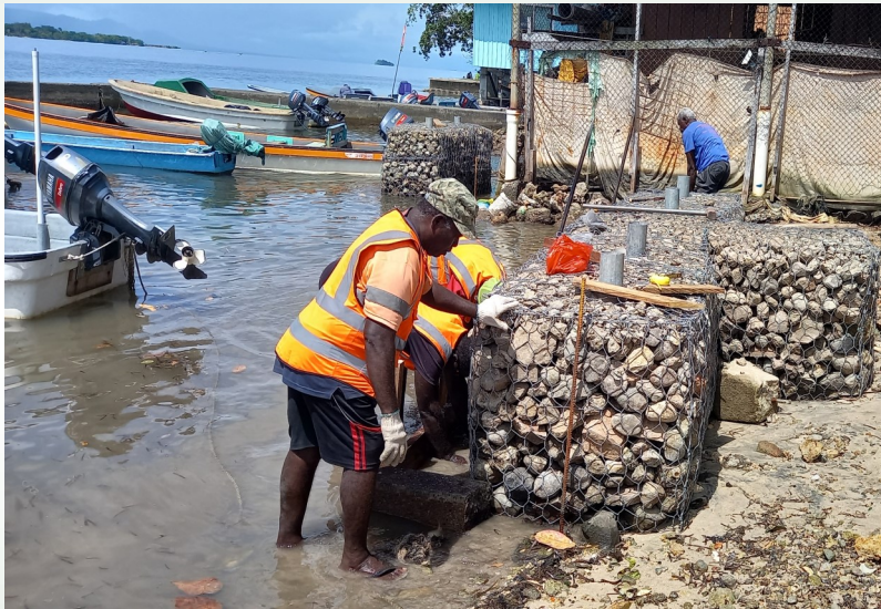
Work on the shoreline protection at Gizo provincial area is progressing well.
