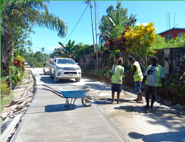
The concrete road at Burinasi to Rurusia almost 80% done. Few more sections to be concrete then it should be fully completed , about 80% done.
