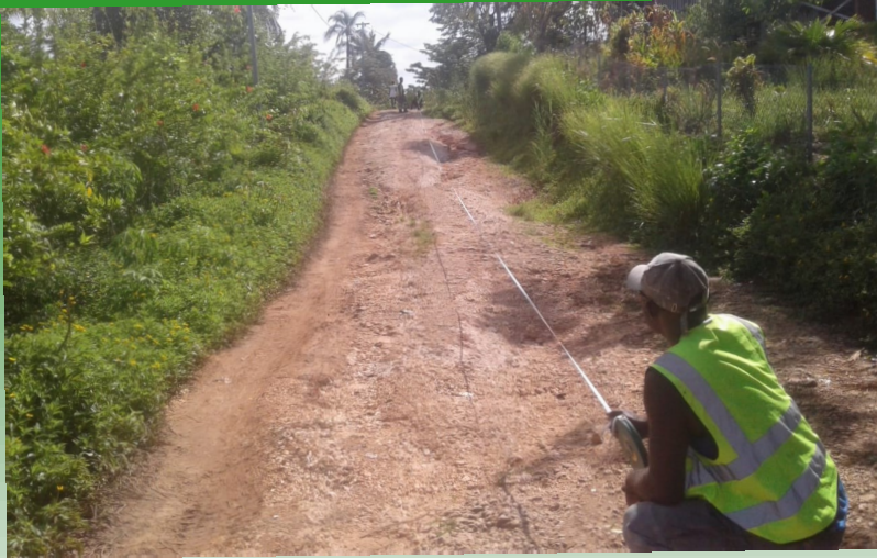
Marking out of the rough section of Jah Mountain road has completed. Next week work will start on concreting the road.
