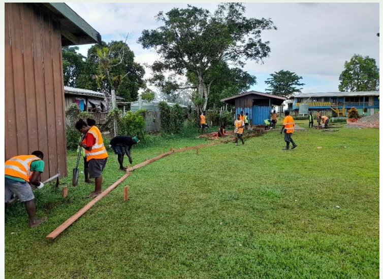
Work is currently going on at Noro for the construction of new footpath around the school.
