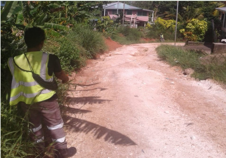
TC road of Gizo will soon be concreted. Marking of the segment to be concrete as been done. Work will start in the coming weeks.
