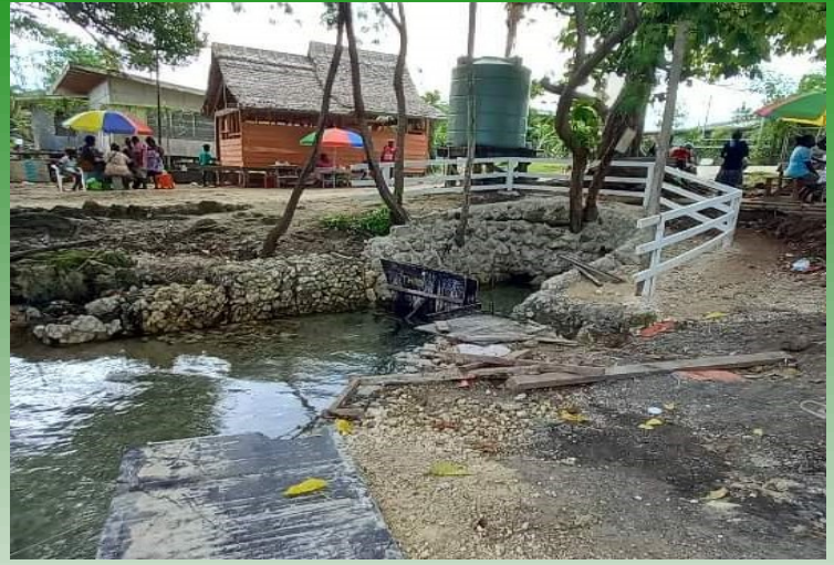
The upgrading of water source at Munda near the market has been completed. The water source will provide water to the ablution blocks at the market .
