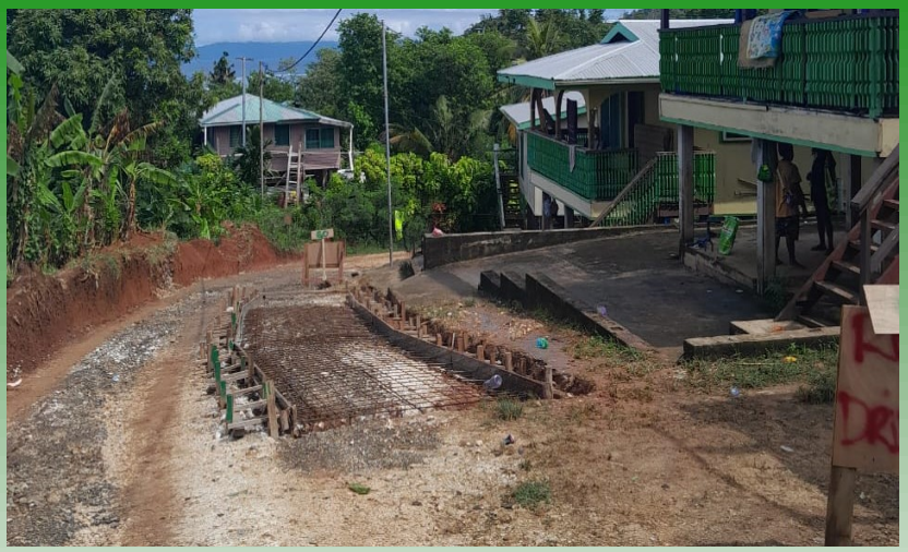
Construction of concrete road in Gizo is progressing well. Concrete pouring will be done this afternoon depending on the weather.
